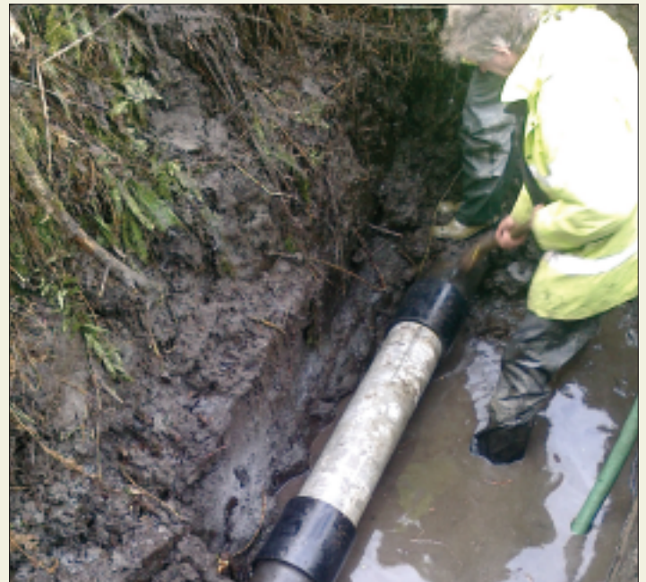
Leak detection and repair is an ongoing process for the staff of Kilmaley-Inagh GWS. However, most leaks are on consumers' premises and not on the mains.
