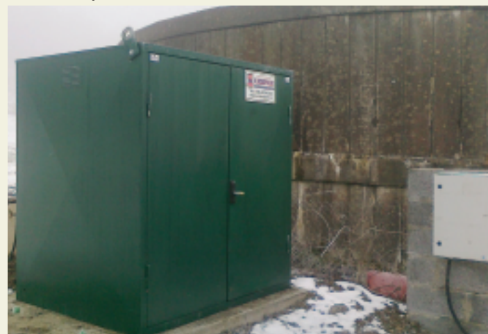
The secondary chlorination station installed at Been reservoir.
