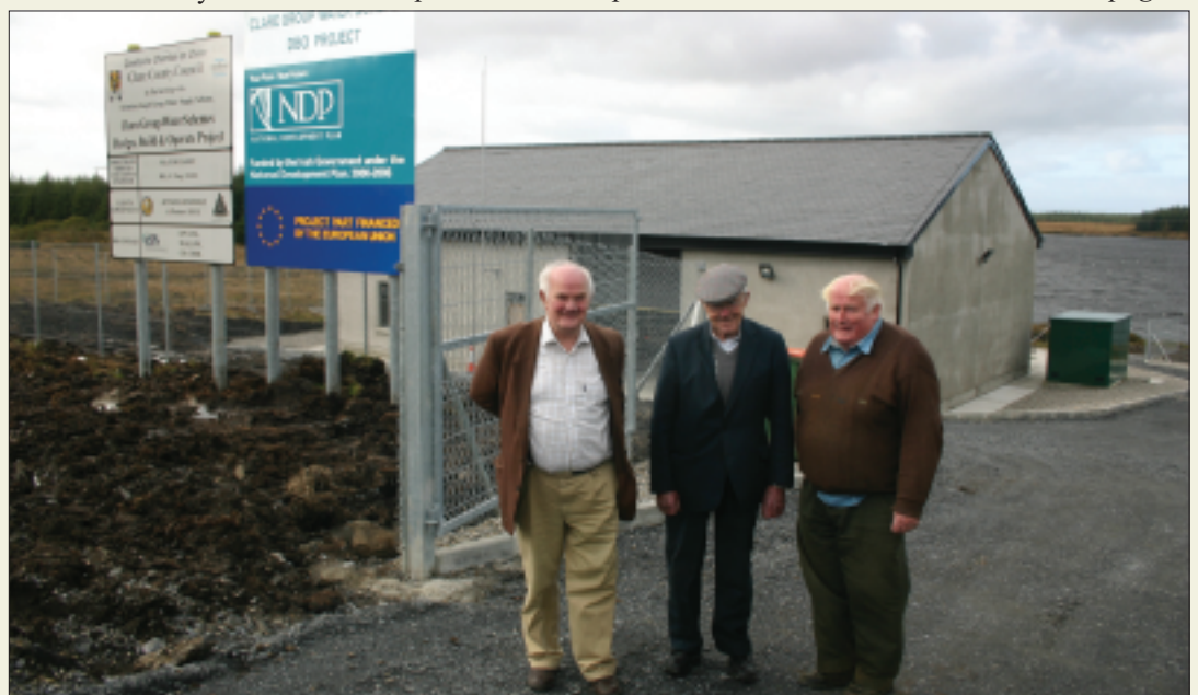
Committee members Tom Burke, Jimmy Meehan and James B. Lynch at the treatment plant following its completion in 2006. Kilmaley-Inagh GWS committee is determined that shortcomings in the plant's operation since then will be fully resolved by the completion of an additional treatment process this year at a cost of €640,000.
