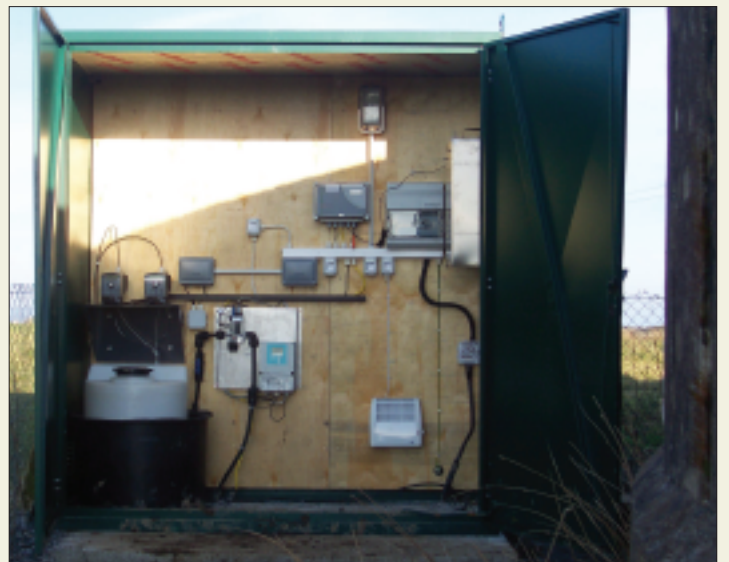
Kilmaley/Inagh GWS water supply is also monitored remotely and secondary chlorination stations, such as the one installed this year at Tullasa (above), ensure that disinfection is maintained to the end of the network.
