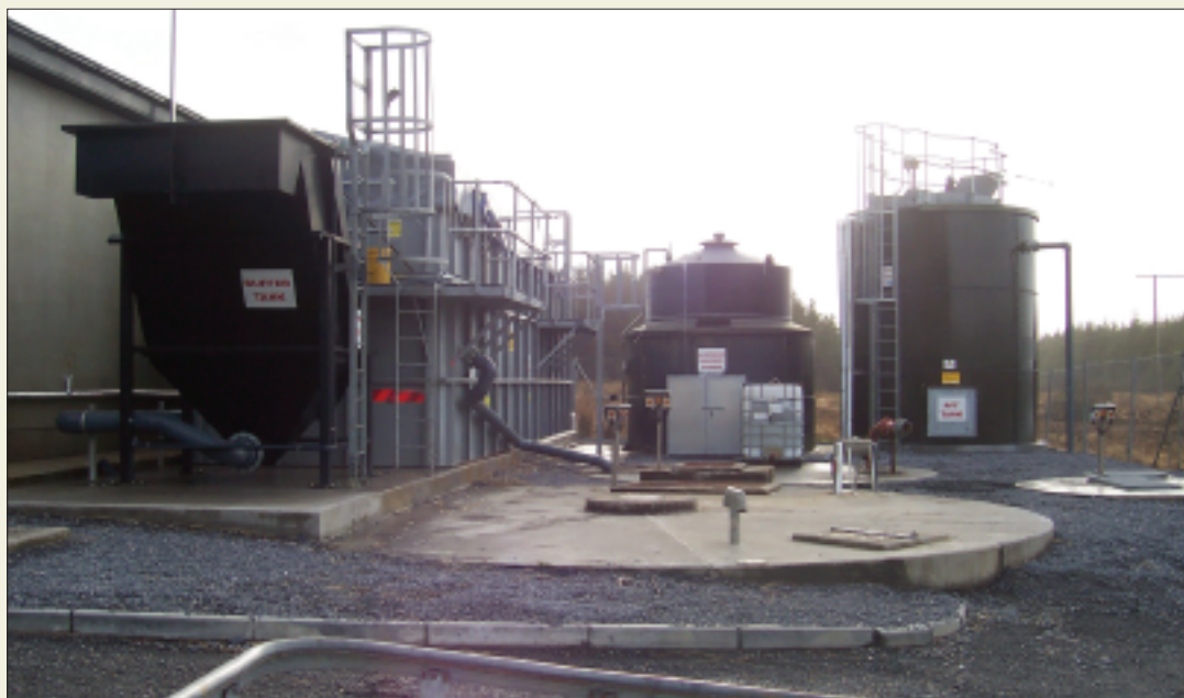
The recently-constructed Dissolved Air Flotation (DAF) plant at Kilmaley-Inagh GWS. This plant removes about 90% of colour and turbidity from our raw water, while a pressure filter process deals with the remainder.
