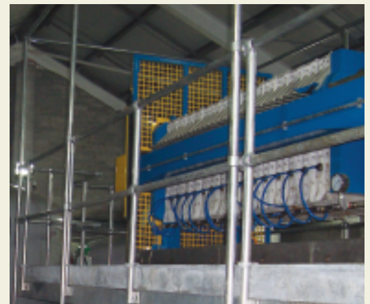
The plate press recently installed in the DBO treatment plant as part of a major upgrade.
